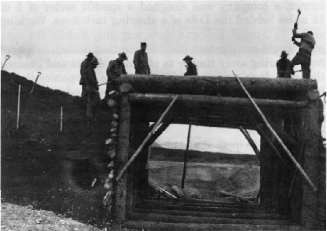
Timber box culverts were used in great numbers along the Alaska Highway. Timber was plentiful and used generously for every possible application.
