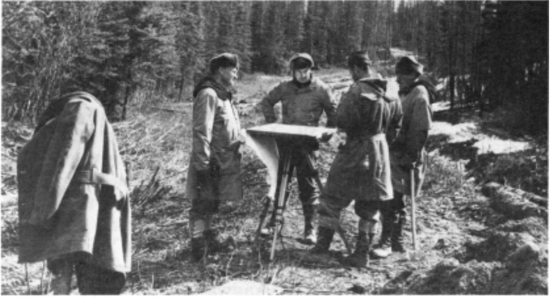
In the northern sector of the Alaska Highway, topographic engineer survey teams work with Public Roads Administration crews to mark locations for the clearing crews.
