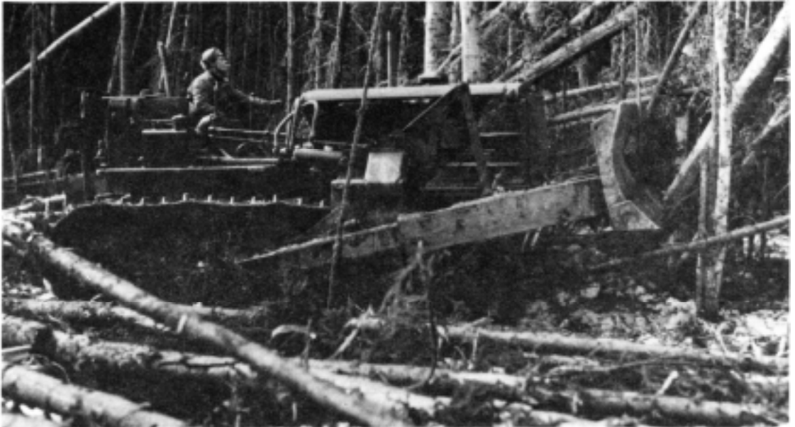
The Caterpillar D-8 bulldozer allowed engineer regiments to clear, cut, fill, and grade the pioneer road faster than had been planned.
